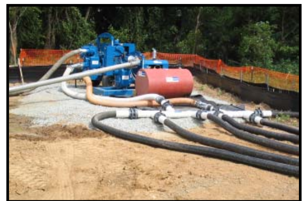
Two Thompson Vacuum Assisted Dry Prime Trash Pumps attached to the manifold used to regulate the suction of the wastewater.
