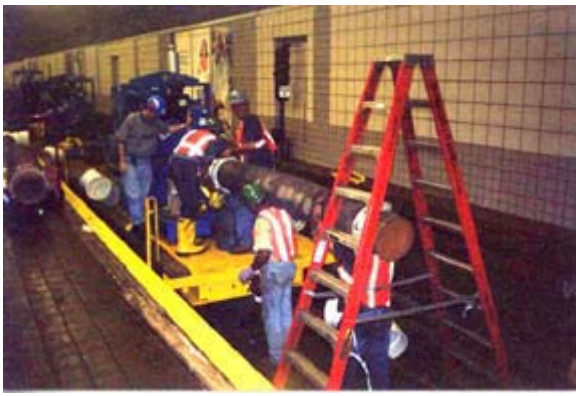
The team comprised of representatives from Thompson Pump, the Port Authority and the contractor sets up the discharge pipe system.
