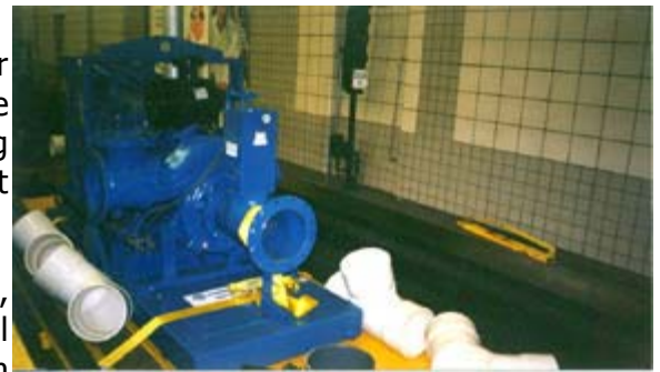
The two 12-inch pumps had to be brought into the tunnel on rail cars.
