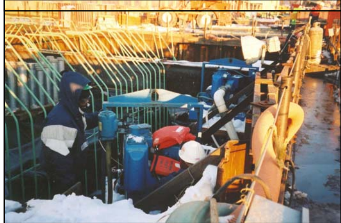
Thompson's service team was on call during the entire concrete pouring process. Pump & Power Equipment provided additional support with immediate parts and service as well.
