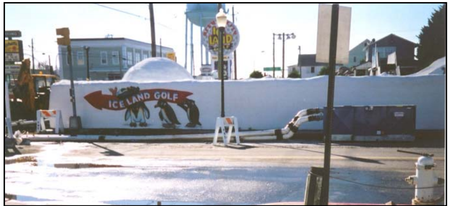
Thompson's Piston Wellpoint Pump with Sound Attenuated enclosure operating near one of the attractions in Ocean City.
