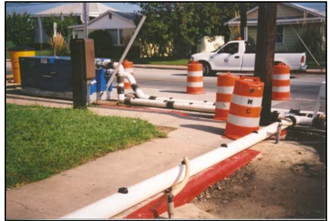
The Thompson Piston Wellpoint Pumps provided sound reduction, efficient fuel consumption and enough power to complete the job before the busy tourist season started.
