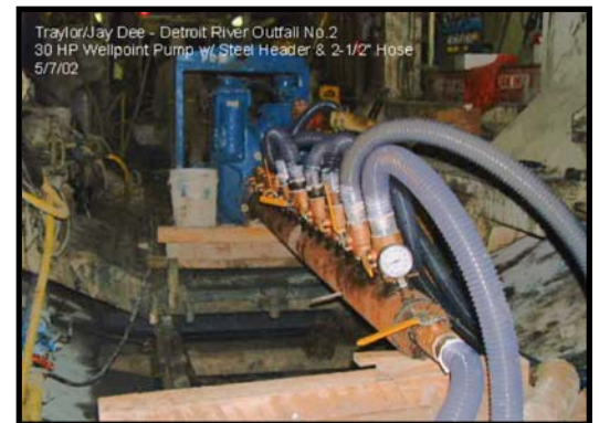
Thompson Pump's 6-inch Dry Prime Vacuum-Assisted Pump removes the water from the tunnel segments.
