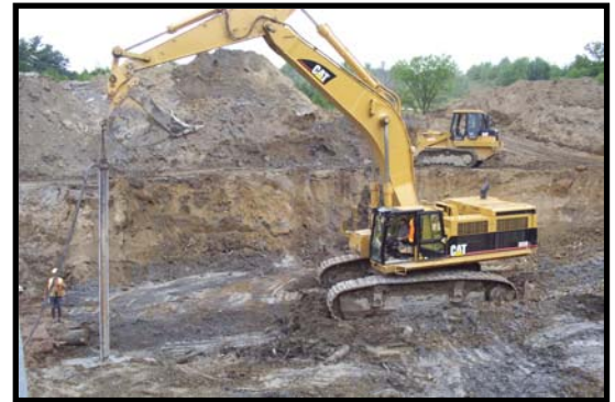
Installing the wellpoints using a punch and casing method is used when the soil conditions indicate that the ground is too hard for self-jetting.
