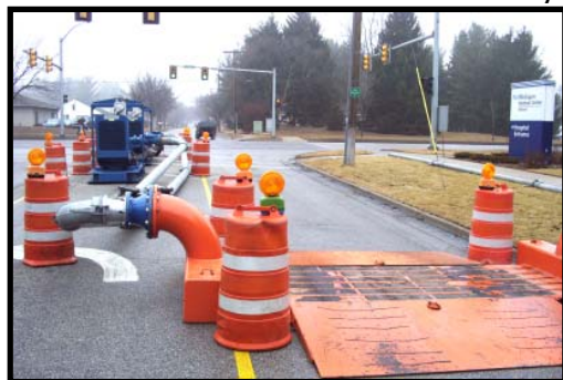
A 12" Road Ramp was required to keep the traffic moving because the bypass was located in front of a local hospital.
