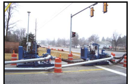
Two Thompson 6-inch Solids Handling High Pressure Pumps were used on the Midland Bypass
