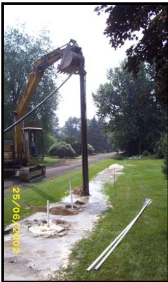
A crane is used to help drive the casing and wellpoint into the ground.
