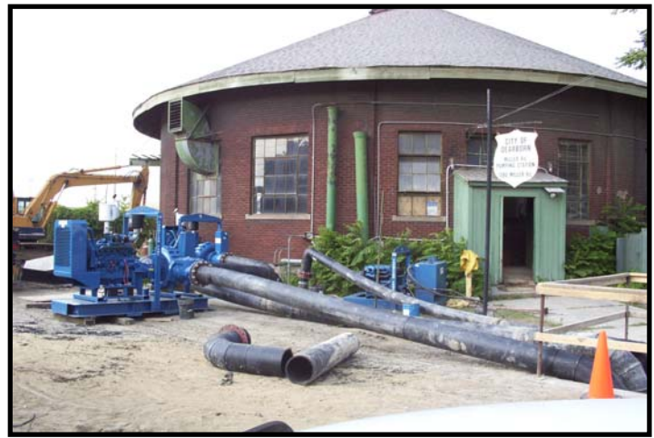
Thompson Pump's 12-inch Solids Handling High Pressure Pumps and 8-inch Hydraulically Driven Submersible Trash Pump on the Miller Road Pump Station.
