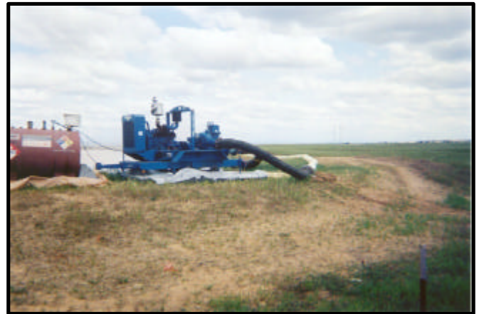
Thompson Pump's 8-inch Solids Handling High Pressure pump was used to handle the water in the storage pond.
