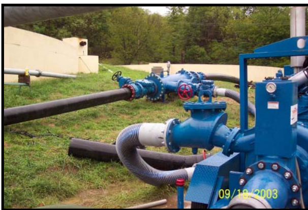
The pump's discharge led into a common manifold and then led on into the force main. The HDPE pipe, being heavier than other types of discharge pipe, and because it is fused rather than connected, eliminated the water hammer concerns.
