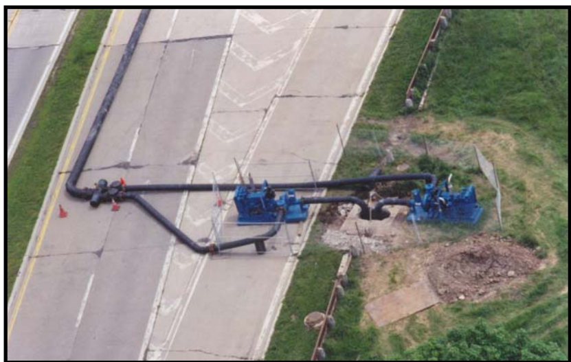
Thompson 12JSC high pressure solids handling pumps
