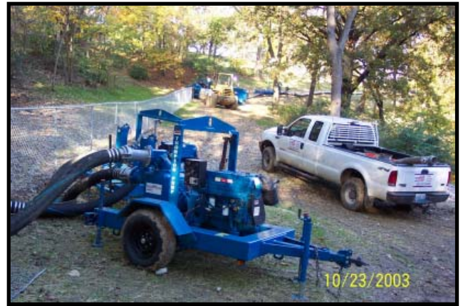
A 6-inch Dry Prime Trash Pump with the ENVIROPRIME ® Priming System was strategically placed at the available manholes before the main bypass in order to divert peaks in flow and to prevent further surcharging.
