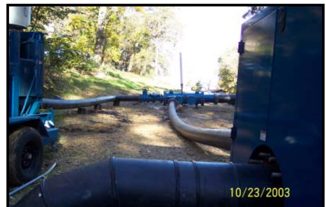
The three pumps discharged through 12" High-Density Polyethylene (HDPE) Pipe and into a common manifold regulated by 12" gate valves.
