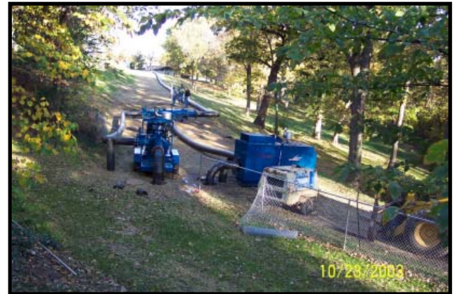
Two Thompson 12-inch Solids Handling High Pressure Pumps and a 6-inch Dry Prime Trash Pump, all with the ENVIROPRIME ® System combat surcharging at Mission Main.
