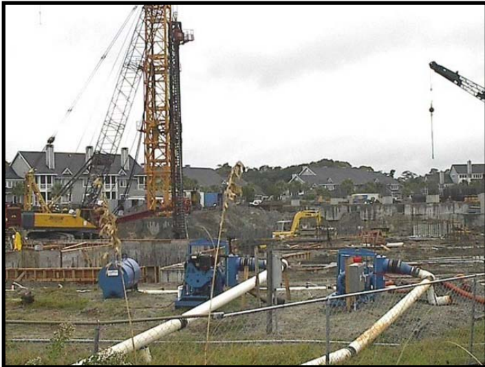
A Thompson electric motor driven 12-inch Rotary Wellpoint Pump was used for the main dewatering with a diesel powered 12-inch Rotary Wellpoint available for standby.
