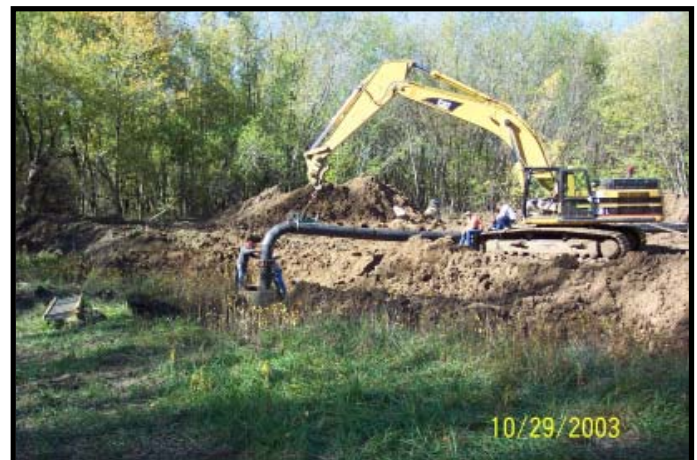
Crews installing the 18" HDPE Pipe discharge into the 120' interceptor 300' away from the bypass operations.
