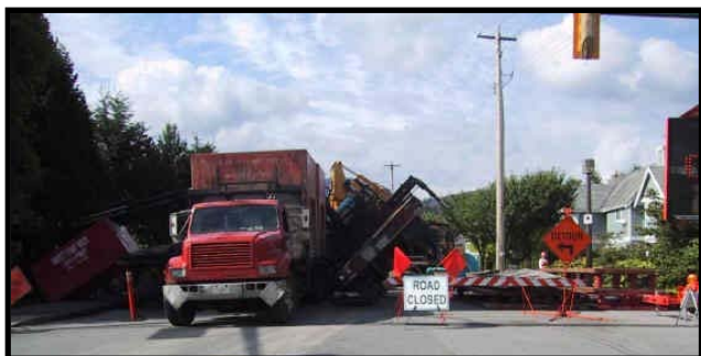
The road was closed to oncoming traffic at the second phase of the bypass to allow construction on the pumping station located nearby.
