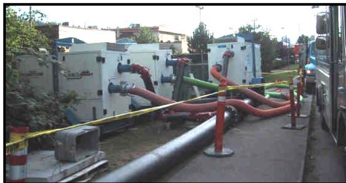
The pumps are installed at the third phase and at the pumping station.
