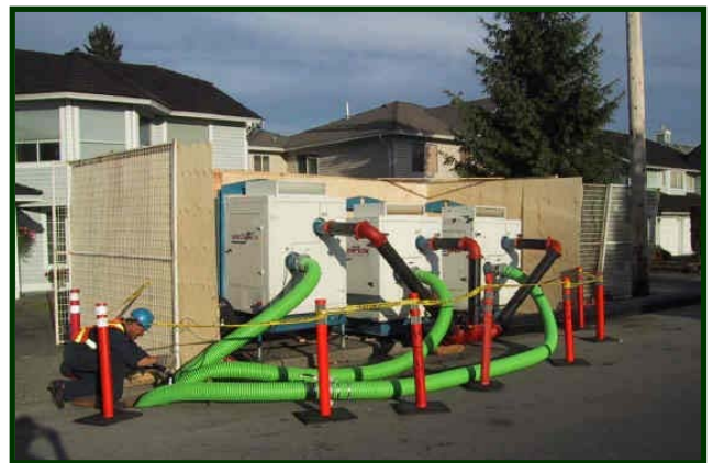
Three of Thompson's 6-inch Dry Prime Compressor-Assisted Open Trash/Sewage Sound Attenuated Silent Knight® Pumps on the first phase of the bypass operation.
