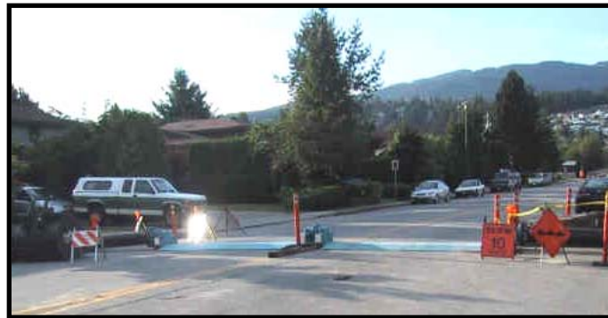
The road ramps installed to direct the discharge from the first phase across the street in line with the Landsdowne Pumping Station.
