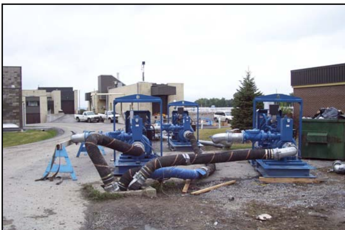
Three Thompson 6-inch Portable Solids Handling High Pressure Jet Pumps are strategically placed around a manhole opening.
