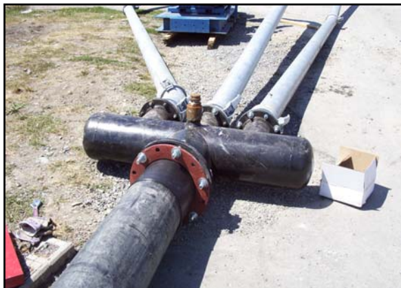
Manifolds, such as above, directed the sewage to discharge points.
