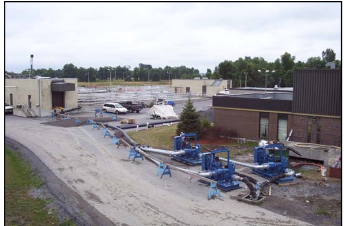
Overview of the first bypass system.
