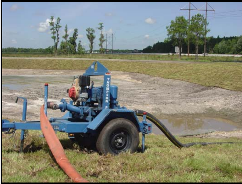
A Thompson Pump Diaphragm Pump dewatering rainwater that collected in an already dewatered pond location. Rain was an issue that had to be dealt with each day. Because the soil was dense in some areas, rainwater could not seep into the ground. New ponds were excavated in order to provide a place for rainwater that landed on the dense soil to collect.
