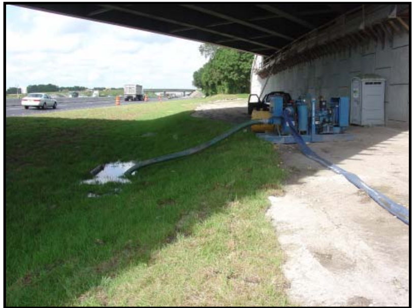
A Thompson Pump 8-inch Vacuum Wellpoint Pump dewatering a stormwater drain under an overpass on Interstate 4 near the Polk County line.
