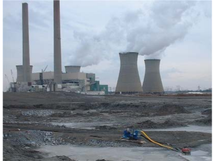
Thompson Pump's 8-inch Dry Prime Open Trash sewage pump dewateres the Power Plant's sinkhole.
