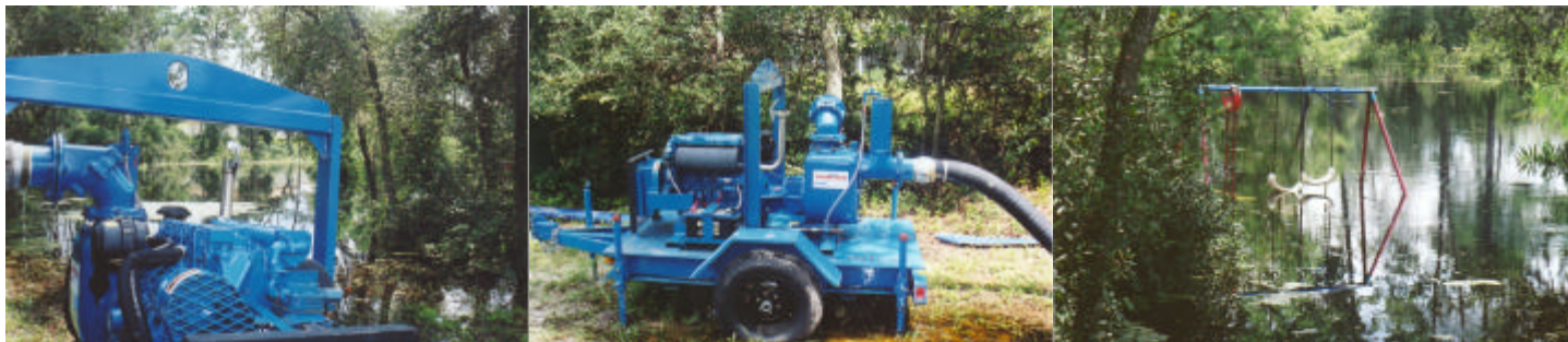
A Thompson Pump ENVIROPRIME® Dry Prime Pump being used to dewater the backyard of a residence. Notice the water level almost comes as high as the bottom of the swing set's swings.
