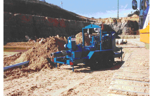
Crews used the surrounding dirt to keep the suction hose secure while the pump was operating. The distance from this platform to the surface was approximately 100-feet.
