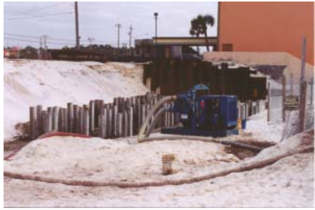
Thompson Pump being used in a piling application in Panama City Beach, Florida.
