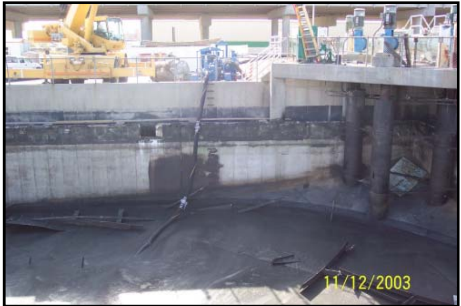
Thompson Pump on the job: pumping out the West Side Treatment Plant's clarifier allowing for much-needed refurbishment of the clarifier.
