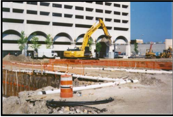
Next to the Parking Garage project, construction was taking place on Bally's/Caesars Transportation Center
