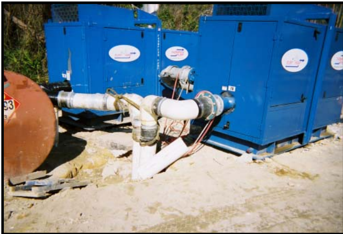
Two 8" Sound Attenuated Solids Handling High Pressure JSC Series pumps with the ENVIOPRIME® Priming System were used in phase one of this bypass project. The pumps were responsible for moving over 2-million gallons of sewage per day.
