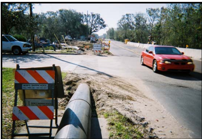
Because HDPE pipe is flexible it can be cut to fit and fixed at angles, driveway crossings were not needed along the road. The contractor cut the roadway to allow the HDPE pipe to be installed underground, and then re-covered the road with a temporary surface. This allowed traffic to move freely while the bypass was in operation.
