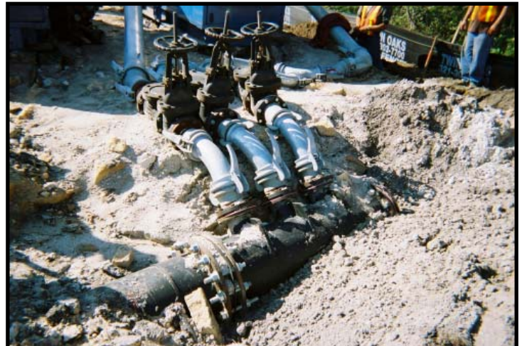
A three-port HDPE (high-density poly-ethylene) manifold, complete with isolating valves, was used to direct the discharge of the two 8JSC pumps, and allowed the customer to remove pumps, if necessary, without disturbing the bypass operation.
