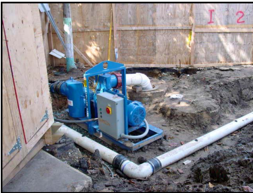
Two 12" Thompson Pump Rotary Wellpoint Pumps were used on the jobsite to remove the groundwater.
