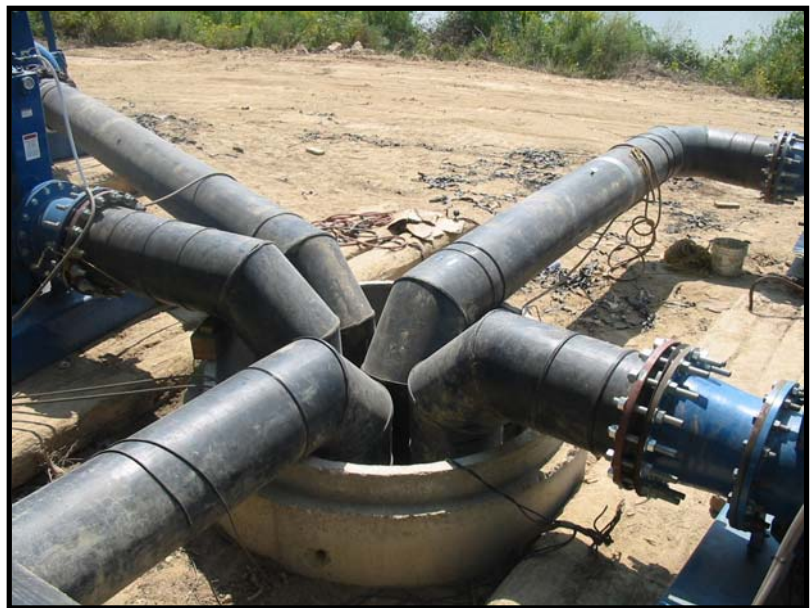
Five HDPE pipe suction lines entering the manhole at the start of the bypass.
