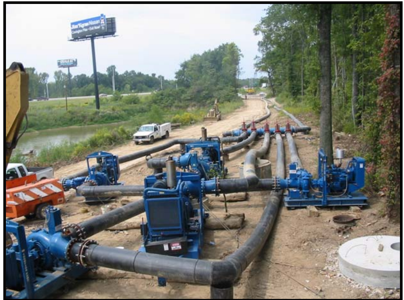
Four 16" and two 12" Compressor-Assisted High Pressure Pumps used for a bypass operated extremely well on White Contracting's largest construction job.
