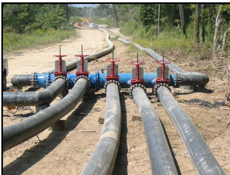
A manifold was used to redirect the discharge from the pumps and reduce the system to two lines which fed into a manhole 750' away from the pumping site.
