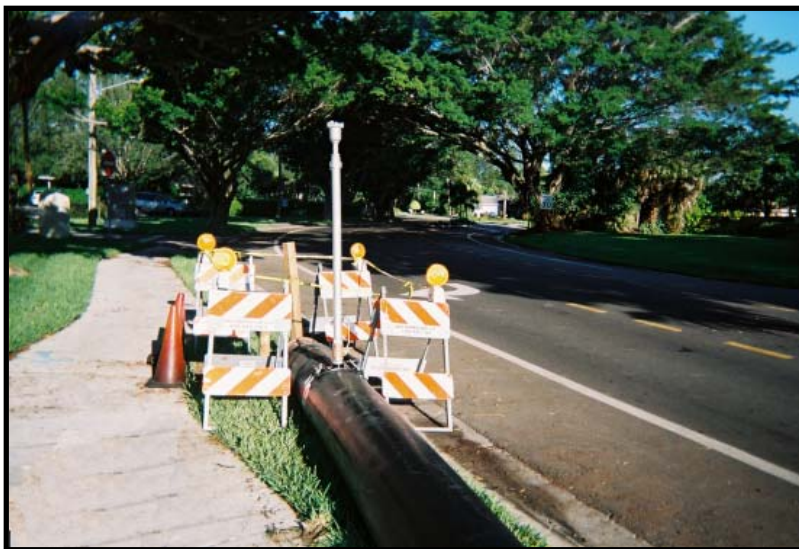
At the final discharge point, an air release valve was used to release air that may be trapped in the system, allowing the pumps to operate more efficiently.
