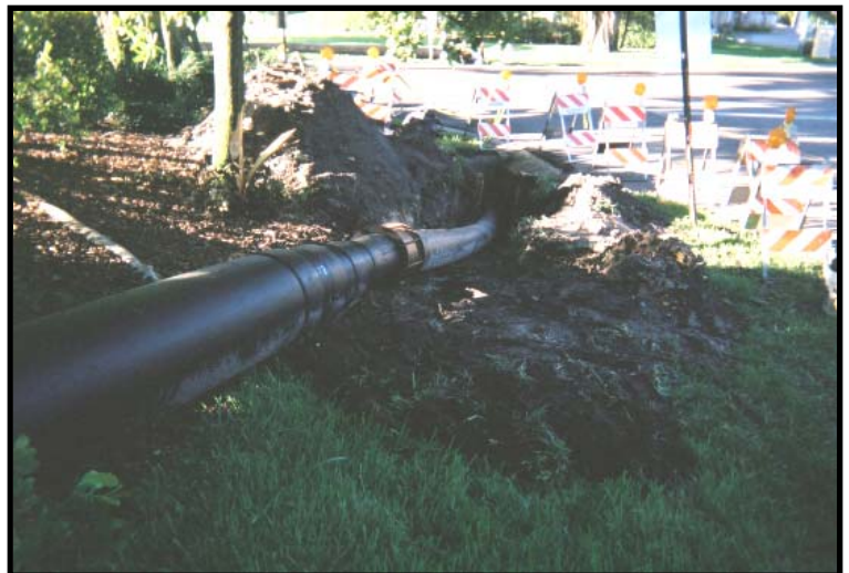
By reducing the size of the discharge pipe from 18" to 12", the discharge line was able to pass through this existing concrete storm drain pipe.
