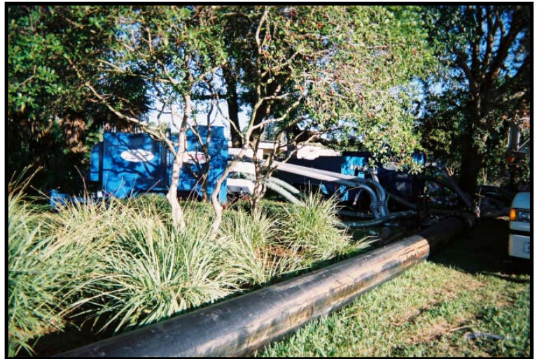
Four Thompson Pump 6" Sound Attenuated Compressor-Assisted Dry Prime Trash Pumps were used for a storm water bypass job in Naples, Florida.
